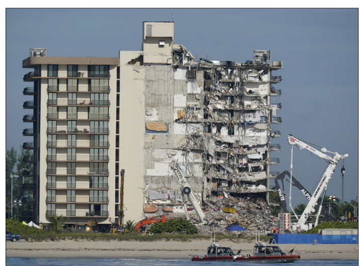
In the aftermath of the Surfside condo collapse in Florida last year, members of the Real Property Law Section analyze ways to avoid such a catastrophe for clients in New York.
